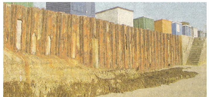
St Helens Duver Wall which clearly shows its poor condition and need of urgent maintenance.
